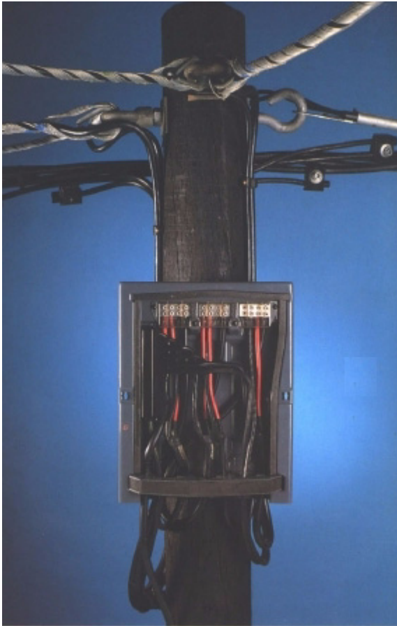
◀ Pole mounted distribution box with a 50mm aerial bundled conductor (ABC) cable connection showing various sizes and types of aerial service connections radiating from it. An 'all-insulated' jointing technique has been employed.
