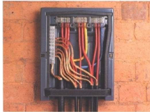
▲ Wall mounted distribution box with incoming 3-core 50mm PVC copper concentric CNE cable and service connections, a mixture of 35mm, 25mm and 16mm PVC copper concentric and hybrid CNE cables (the insulated cover over the neutral has been removed to show the full details).
