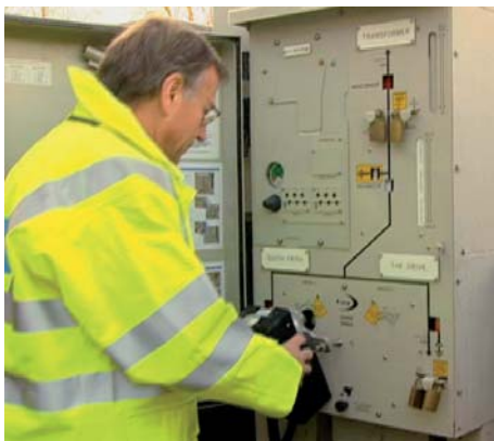
Automated Ground Mounted Ring Main Unit
