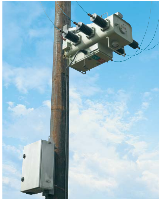
Automated Pole Mounted Load Break Switch
